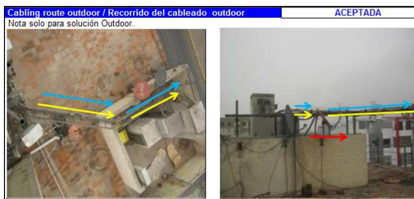
Figura 46. Cableado de Outdoor a Indoor.
